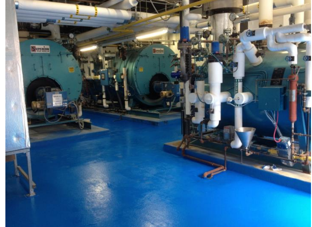
FIGURE 5: New Steam Boilers
